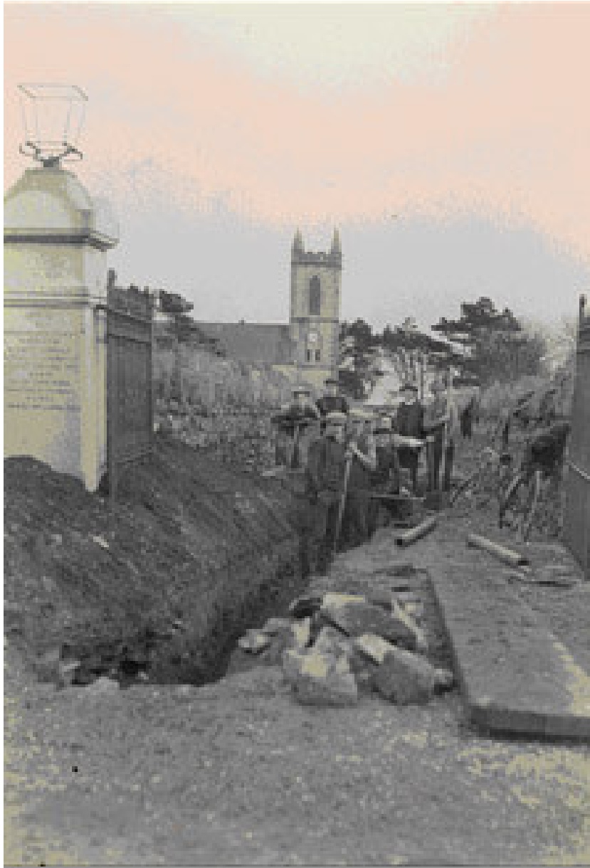
Plate Three: Photograph in possession of Kilhorne Church showing excavation of trench to accommodate water pipe (1932). The photograph depicts Sammy Heaney, Willie Cousins, Rev. T.H.Lyons, Archie Gordon (rear) and John Reidy, Alex Orr, James Gibson, Jim Annett, Ernie Mooney, Hugh Bell (front row). Photograph kindly supplied by the Reverend William Press.
